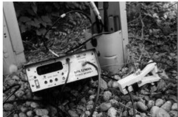
Photo 1. Sheath current induction test at a tap
